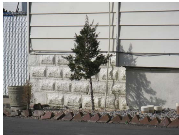
The original home was made of these unique building blocks, most of which are now covered with siding.
